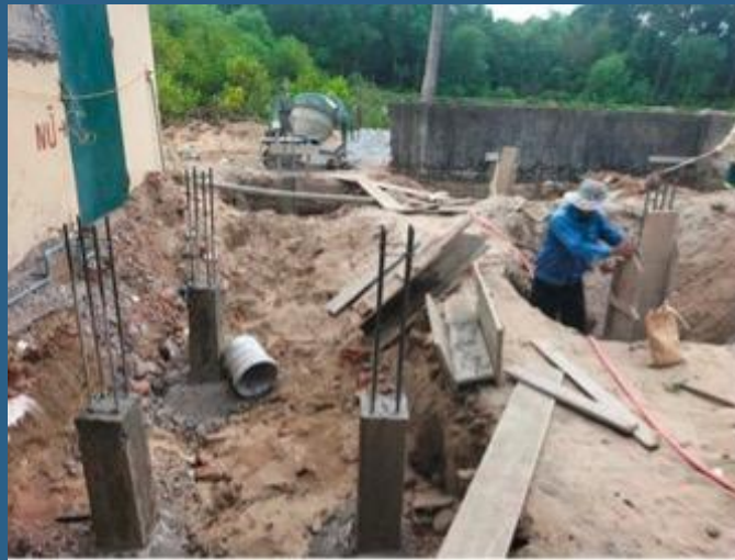
Workers prepare support columns before pouring the foundation for the new restroom.
