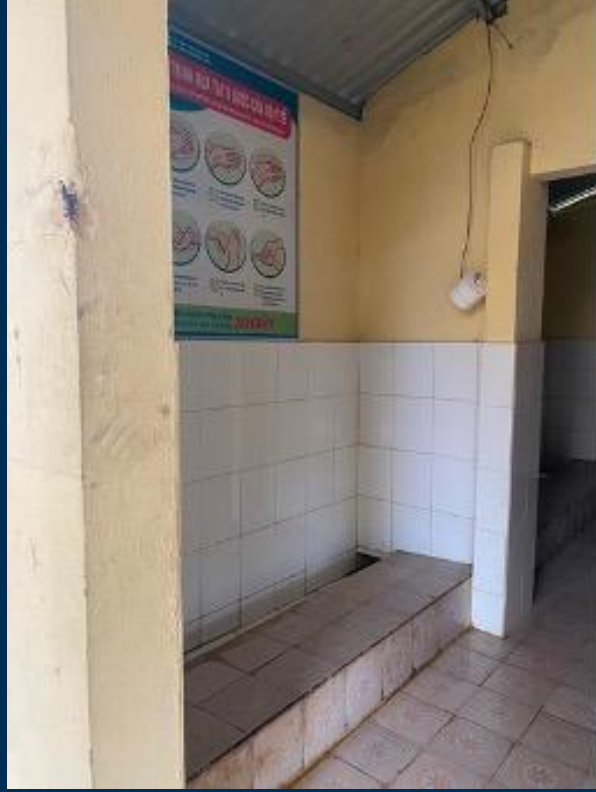
The old restrooms have become outdated, unhealthy, and inadequate.
